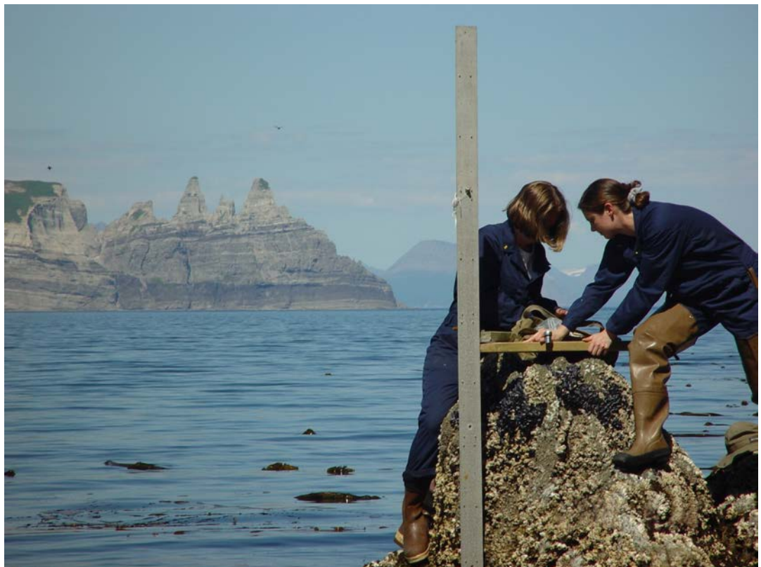
Installing a tide gage near Castle Cape, Alaska – June 25, 2014 Image Credit: Personnel of NOAA Ship RAINIER (NOAA's Historic Coast & Geodetic Survey (C&GS) Collection)
